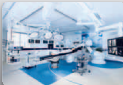
The greatest advantage with the so-called Hybrid OR is that it offers the opportunity to combine radiography possibilities in connection with surgical procedures.
