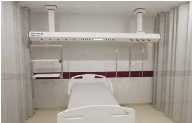
Rack and pole solution.
